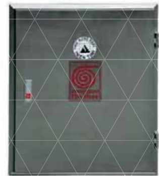
▶ Fire Hose Reel
