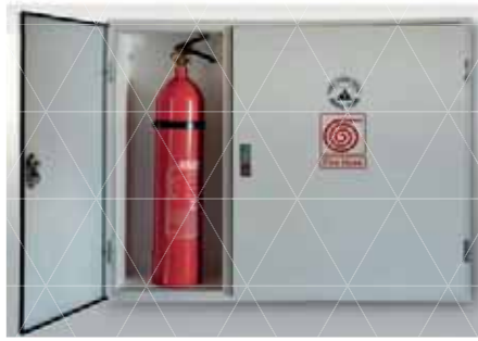
▶ Extinguisher Fire Box
