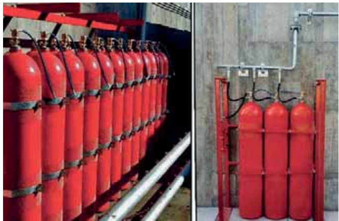
Inert Gas Suppression System (IG System) ◀
